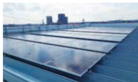
Solar power generation panels installed on the rooftop of Fujimi Store in Kariya City, Aichi Prefecture
