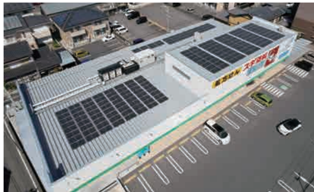
Solar power generation panels installed on a store roof
