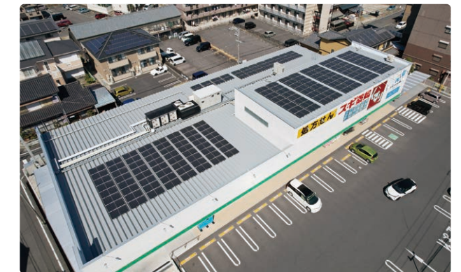
Solar panels installed on a store rooftop
